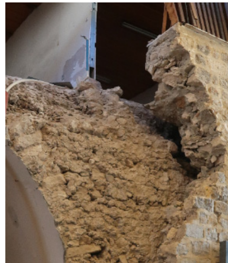
Damaged state of a rubble-stone masonry wall
