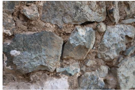
Poor earth mortar
