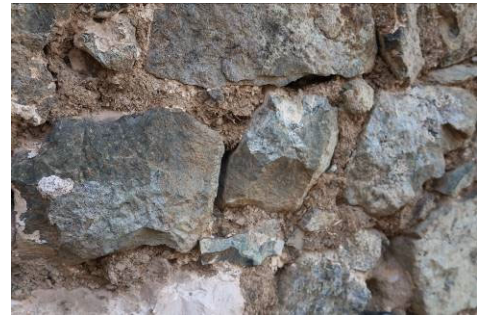
Poor earth mortar
